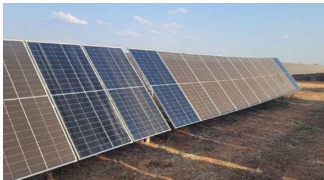
Figure 63 – Example of dirty PV modules and clean modules
