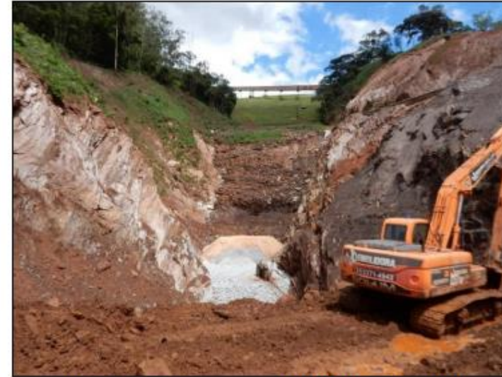
Figure 3. Eroded Toe at Germano Main Dam (March 15, 2016)
