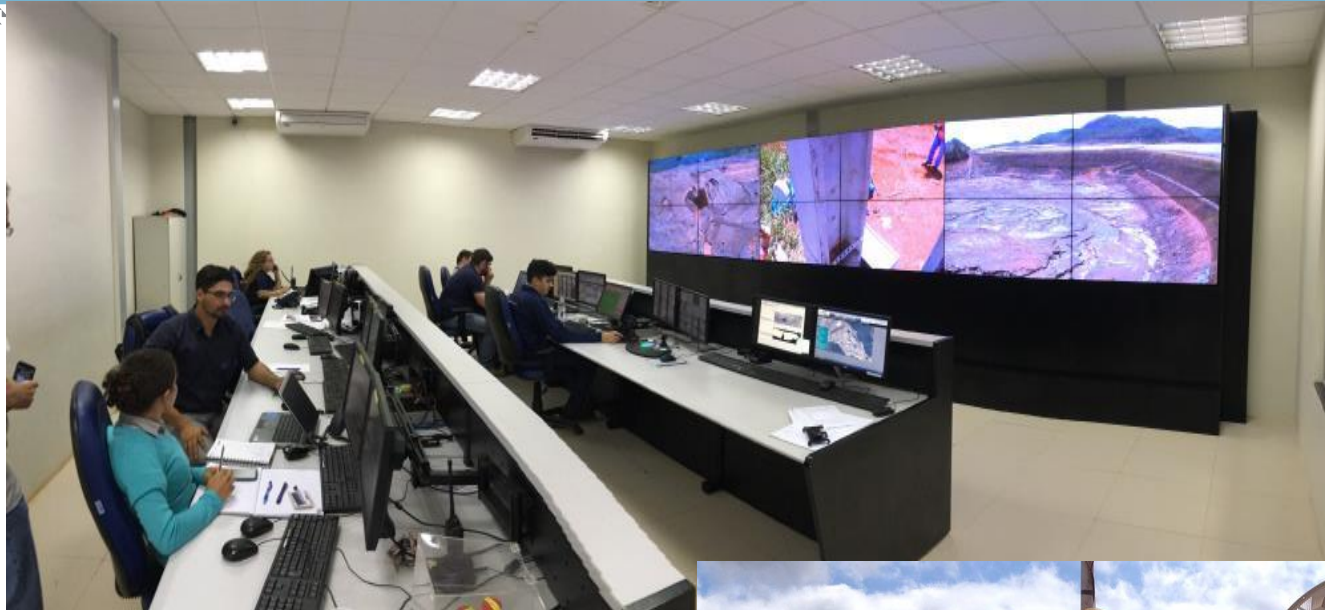
Samarco monitoring control room
