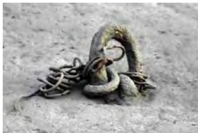
Figure 40. Mooring ring embedded in the stone Source: ANDRADE LIMA, 2013, p. 55
