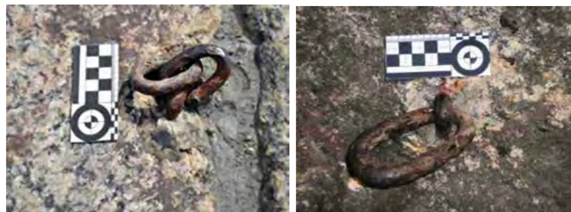
Figure 41: Ferrous metal mooring ring exposed to weathering attached near the edge of the stonework
