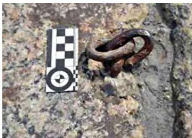
Photo 32 - Ferrous metal mooring ring exposed to weathering attached near the edge of the stonework. Source: ANDRADE LIMA, 2013
