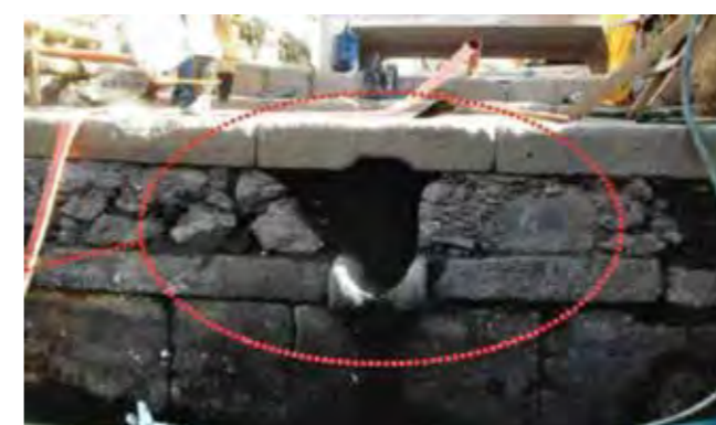
Photo 24 - Drain spout set in (hewn) flagstones of Empress’s Wharf. Source: Ibid., p. 36
