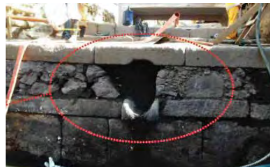
Figure 30. Drain spout set in (hewn) flagstones of Empress's Wharf. Source: Ibid., p. 36
