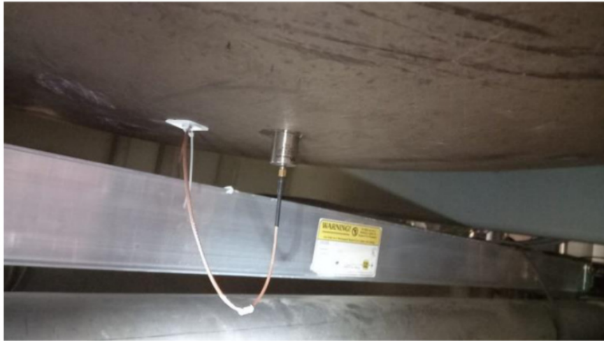
Figure 10.2 - Installed accelerometer installed at the LLO Corner Station.
