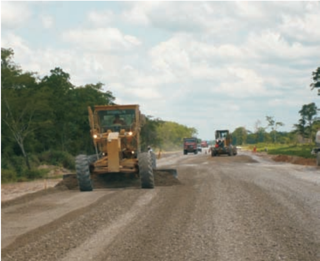
Workmanships of the Highway El Cármen – Arroyo Concepción, Bioceánico Corridor, in Bolivia
