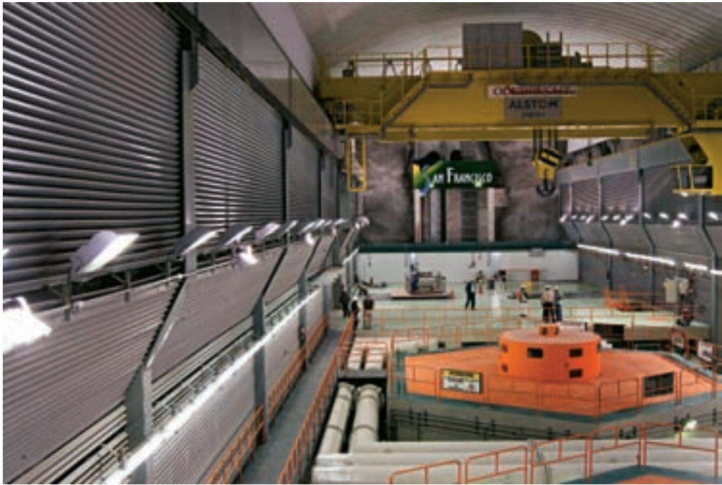
San Francisco Hydroelectric Power Plant in Ecuador
