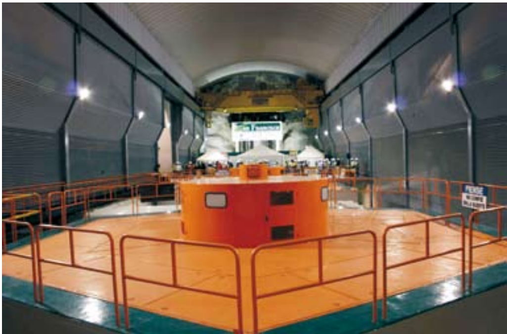
San Francisco power plant (Ecuador)
