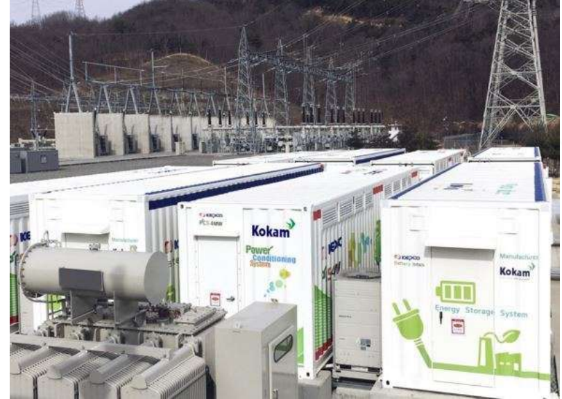
Kokam 56 MW Energy Storage at South Korean
