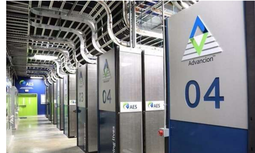
AES Northern Ireland's 10 MW (of 100 MW) BESS
