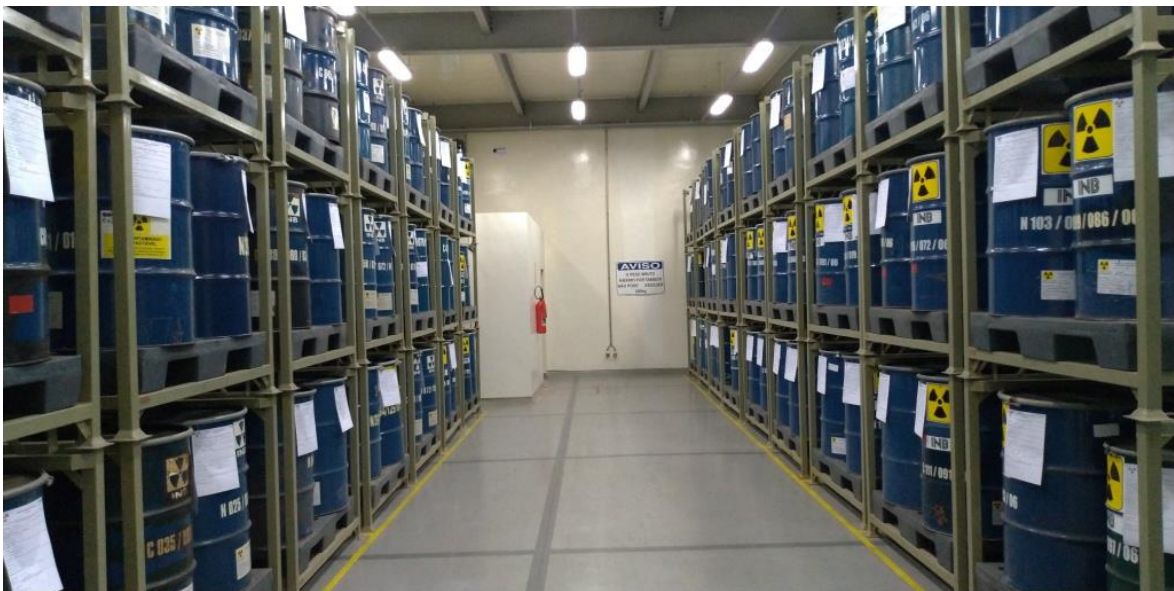
Figure D.1 – Low-level waste storage facility (DIRBA) at FCN
