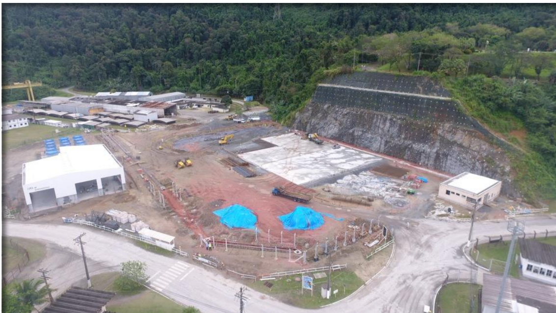
Figure G.4 - Actual Photo of the UAS Facility Construction - September 24 th of 2020
