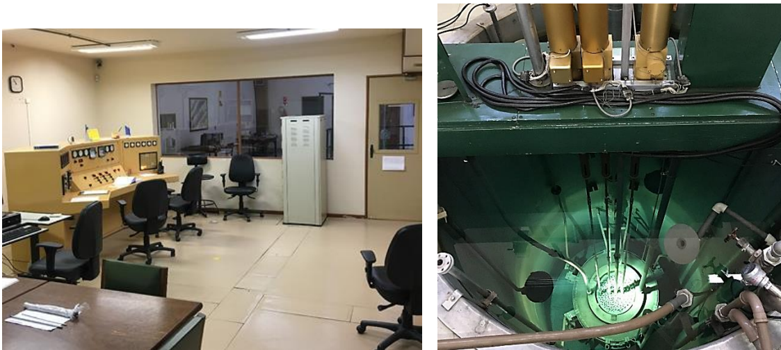
Figure 7 - IPR-R1 – Control Room and Reactor Pool
