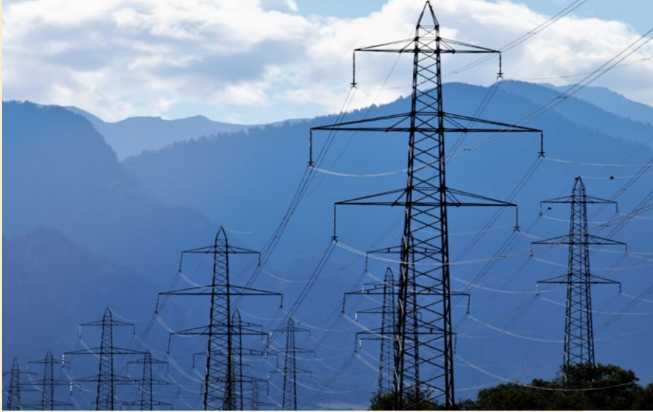
Figure 8 – Electricity supply capacity is a financial variable to be considered in the total cost of ownership of electric buses
