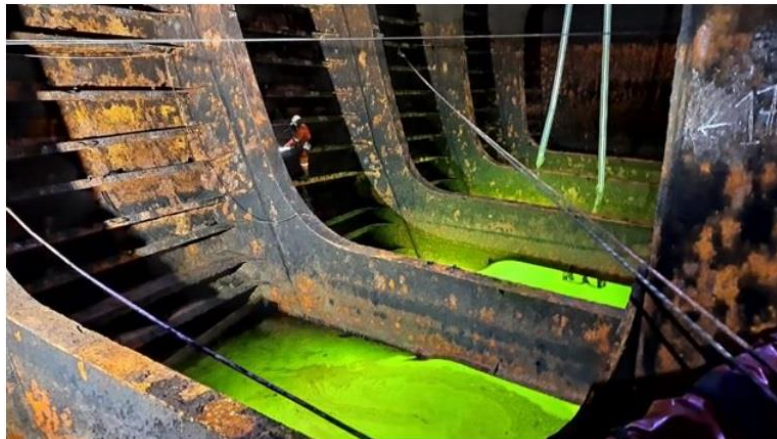
Figure 1 - FPSO hull bottom after tank structural failure.
