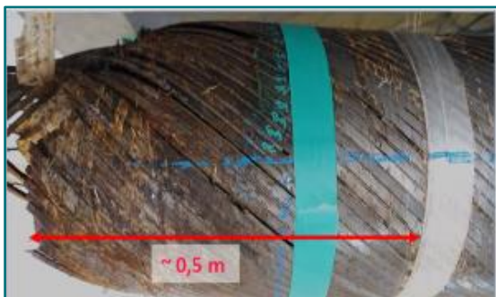
Figure 5 – Severe corrosion of the tensile armour at the end of ruptured riser section (~0,5m)
