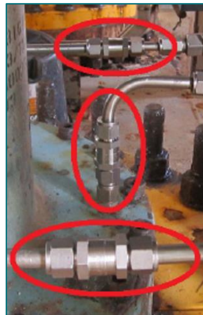
Figure 6 – GRVs installed on the riser annulus vent system lines after the incident
