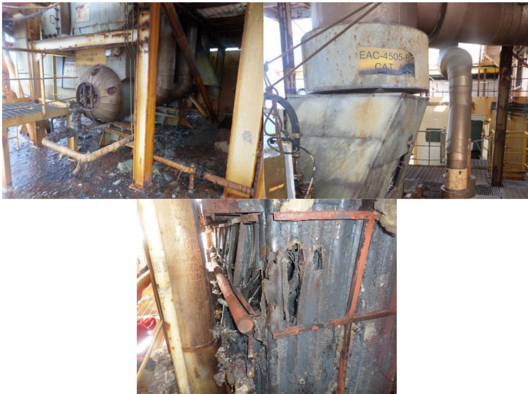
Images of the damaged boiler.
